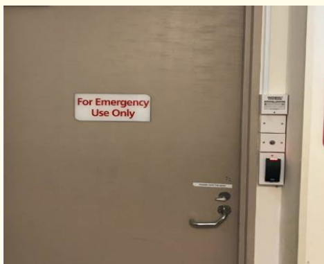
Figure 4: Showing double sided card access from inside and an emergency break glass feature.
